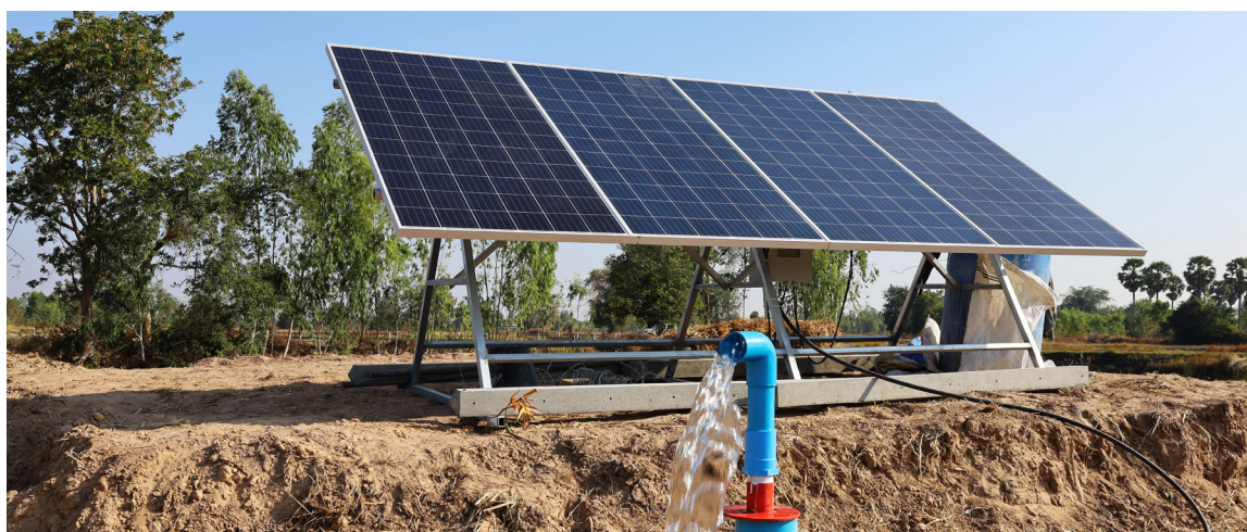
Solar powered irrigation system. Source: Shutterstock.
