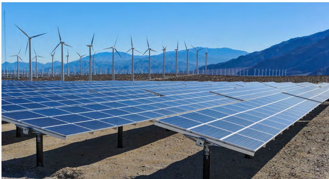
Hybrid power plant at Palm Springs, California, with solar PV and wind turbines. Source: Shutterstock.
