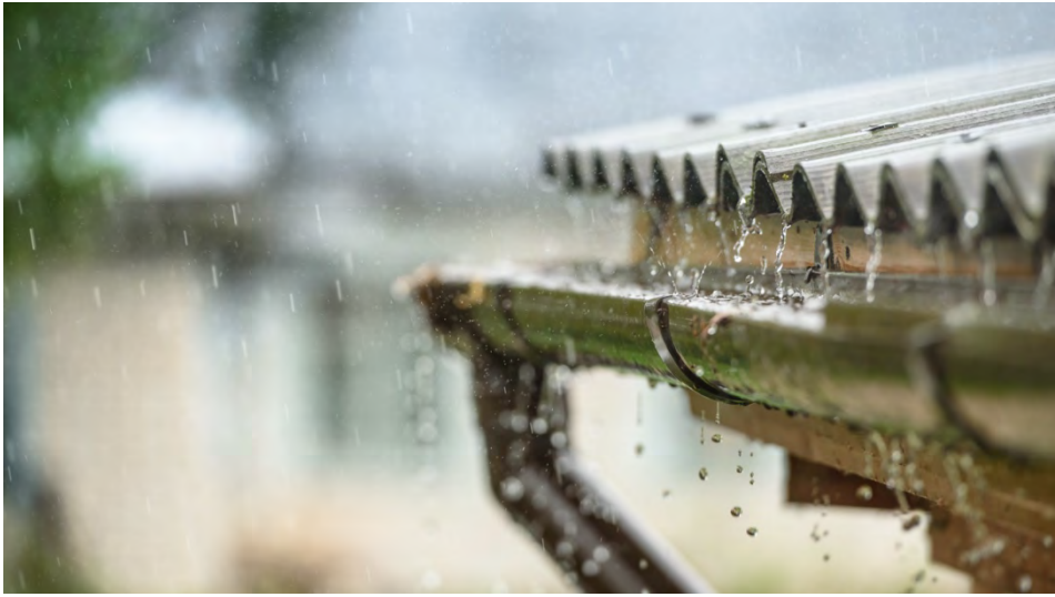
Rainwater harvesting. Source: Shutterstock.
