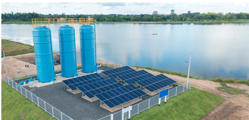
Solar powered water pumping station. Source: Shutterstock.
